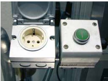
Power supply in the work cage
